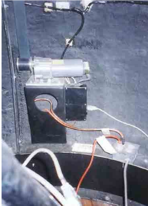
Figure 6: Observatory Dome Control Box and South Side Motor
